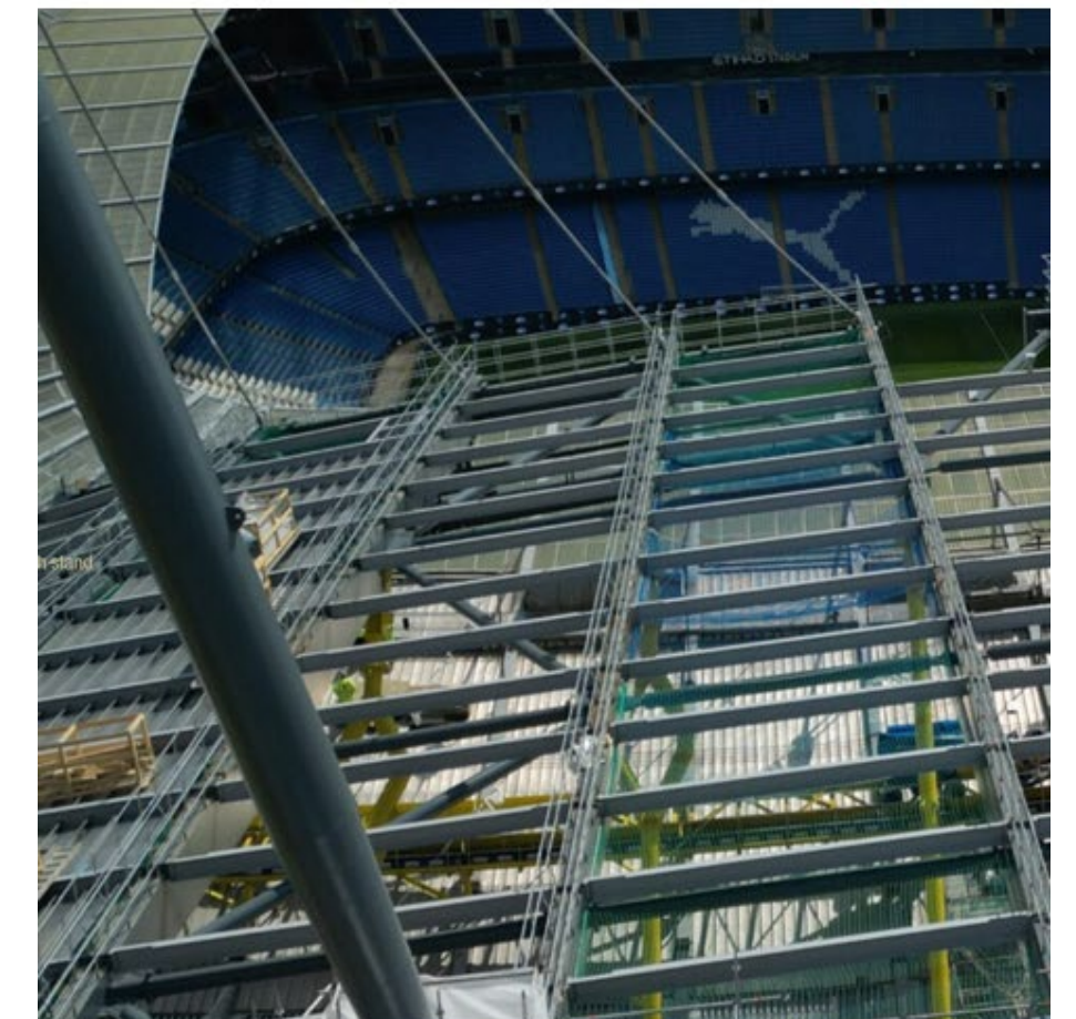
Locally manufactured Steel at the heart of Manchester City's new North Stand, Entertainment District & Hotel project (Sisk)
